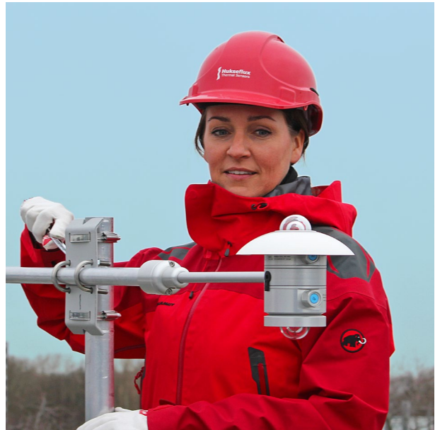
Figure 6 installation of AMF02 albedometer mounting kit and two SR20 pyranometers, mounted with ALF01 levelling fixture on a crossarm with crossarm bracket CMF01.
